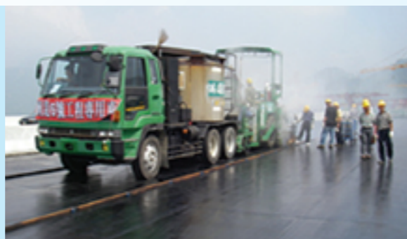
圖15：橋面鋼床板Guss鋪築施工 Fig. 15: Guss-asphalt paving of a steel plate bridge deck
